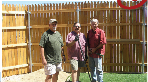
David Thurston, Larry Singleton and Jim Shelburne install grass in the newly finished courtyard at PPTH.
